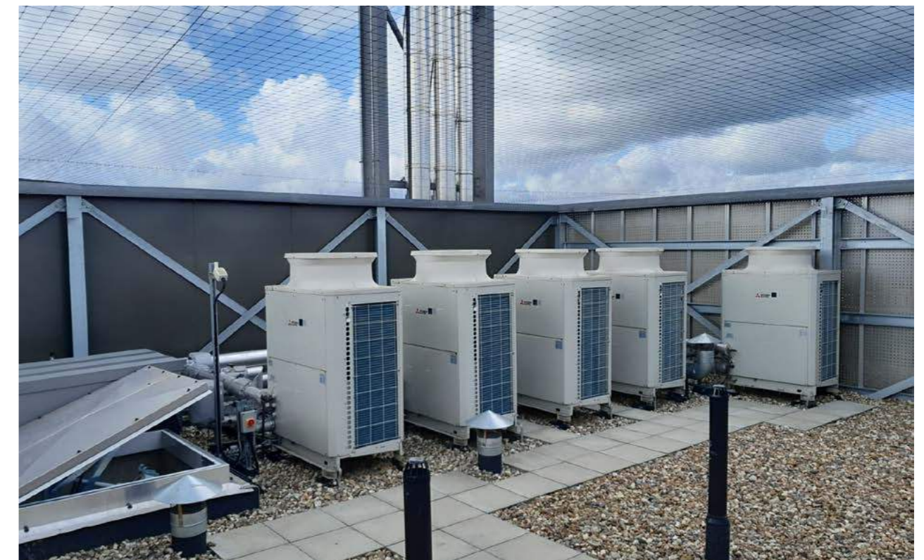
Air source heat pumps at Canalside, Sheerwater
