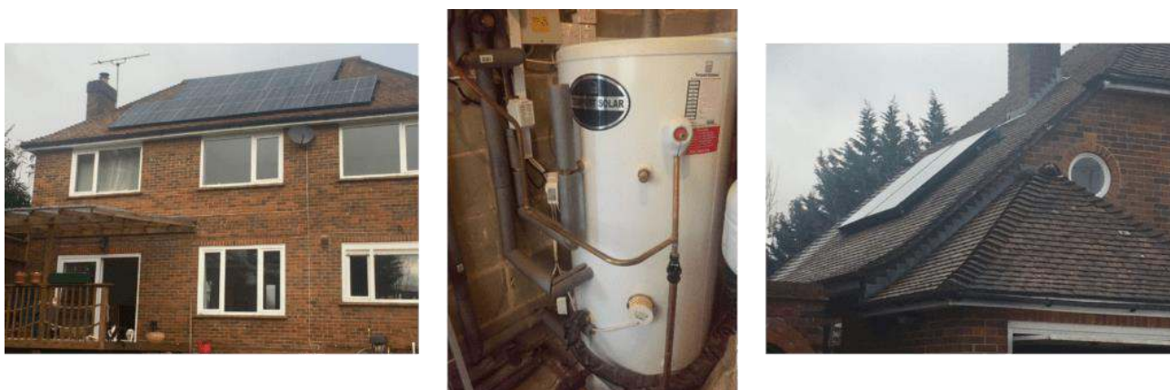
Figure 2: Example of one grant recipient. Left: A ten panel 4kW solar photovoltaic system. Centre: The new solar hot water tank, to store the solar generated hot water. Right: A double panel, flat plate solar thermal collector. Renewables were complemented by cavity wall and loft insulation.
